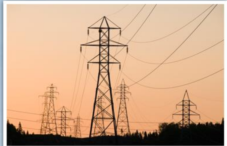
735 kV lines near the 5 616MW Robert-Bourassa generating station
